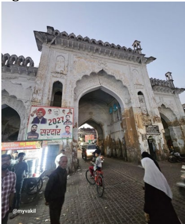
Figure 5 The damaged stucco on Chhota Imambara Gate
